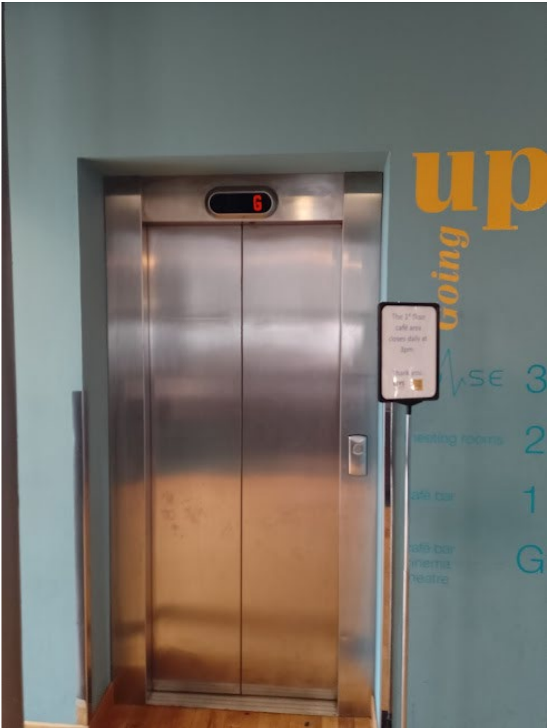
Lift gives access to all floors
