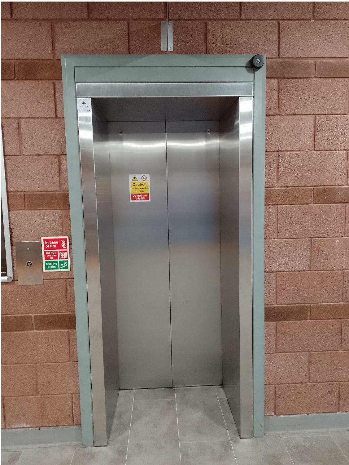
A lift give access to upper and lower levels
